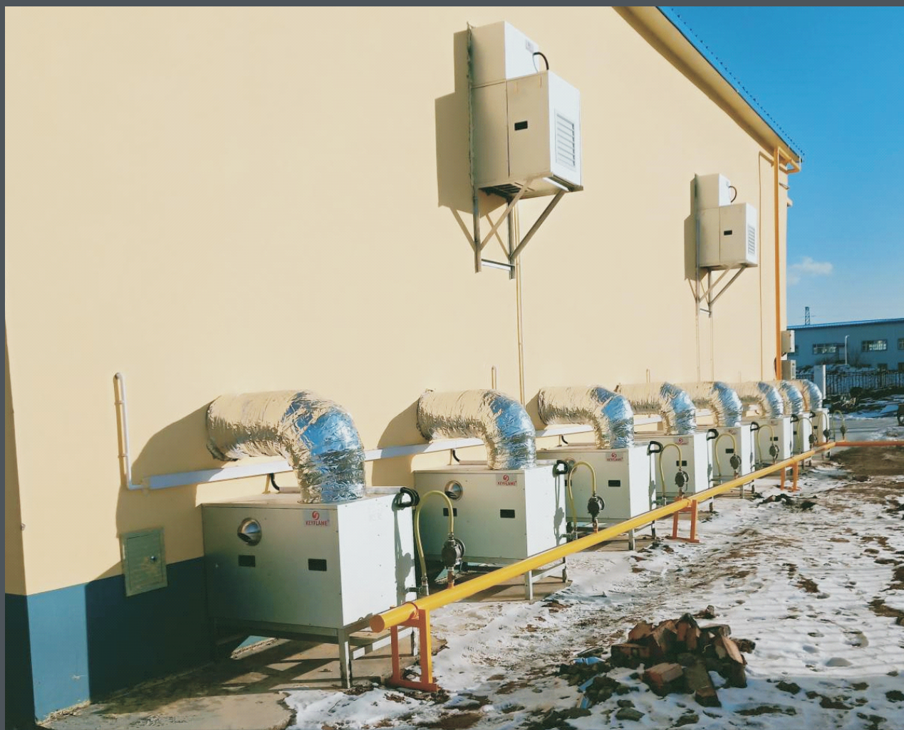
Dryer unit and heat recovery dehumidification device outside the drying room
